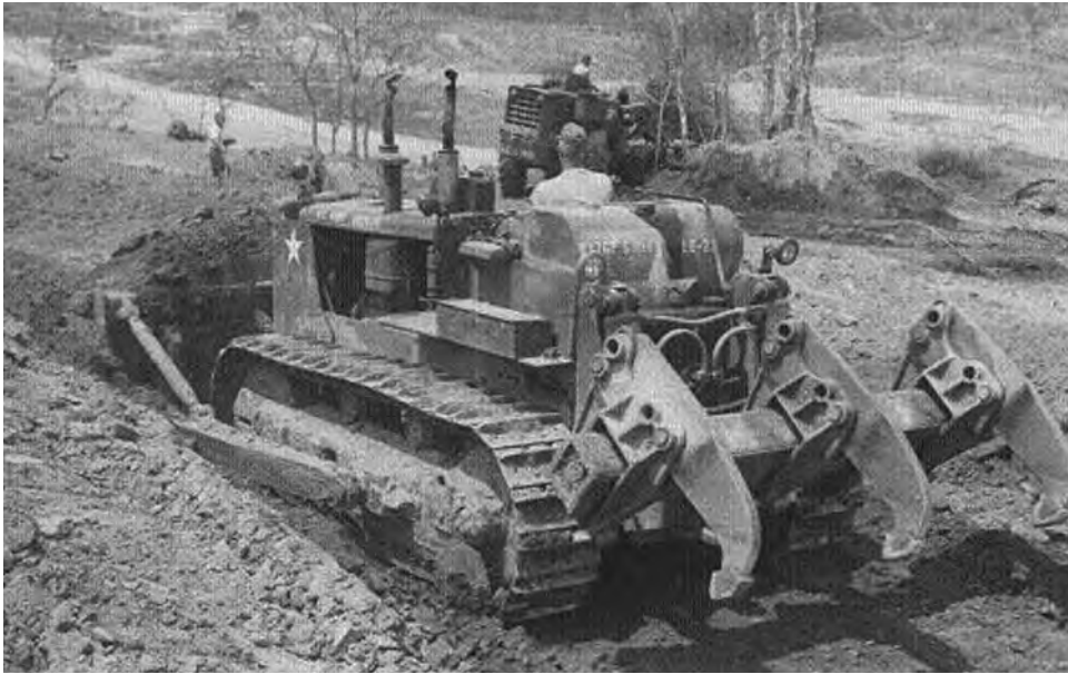
Heavy-duty equipment such as this bulldozer from the 70th Engineer Battalion was used to build roads at the 1st Cavalry Division's Camp Radcliff.
